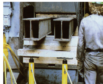
Replacing adjustment rolls under a fly-over with RR cylinders, for controlled lifting and lowering.
